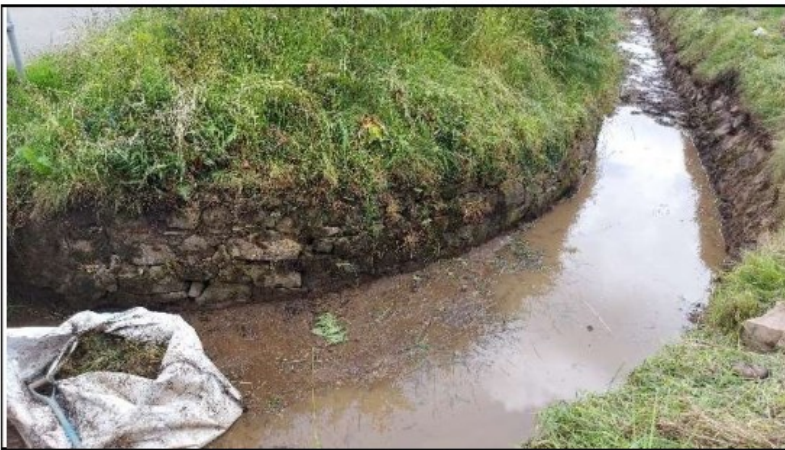
Photo 1: Spillway bend just downstream of bridge. Note this is low spot and is holding water.
