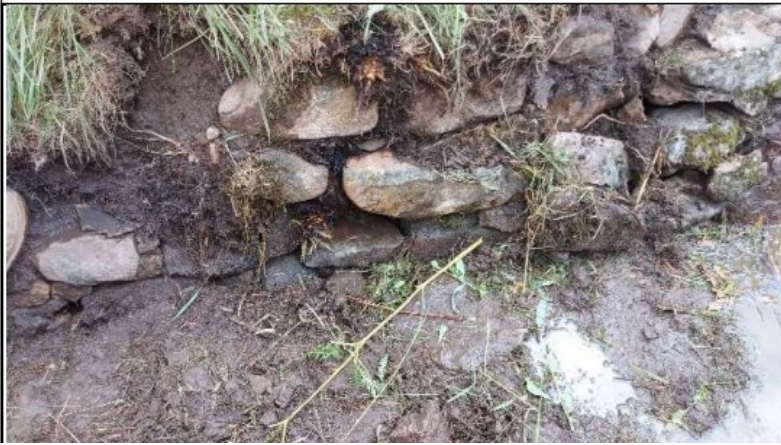
Photo 4: Poor condition on masonry on right hand side of spillway channel.
